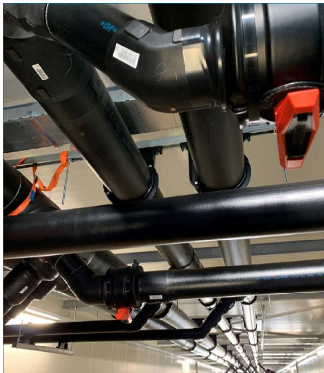
COOL-FIT 4.0 en 2.0 in corridor
